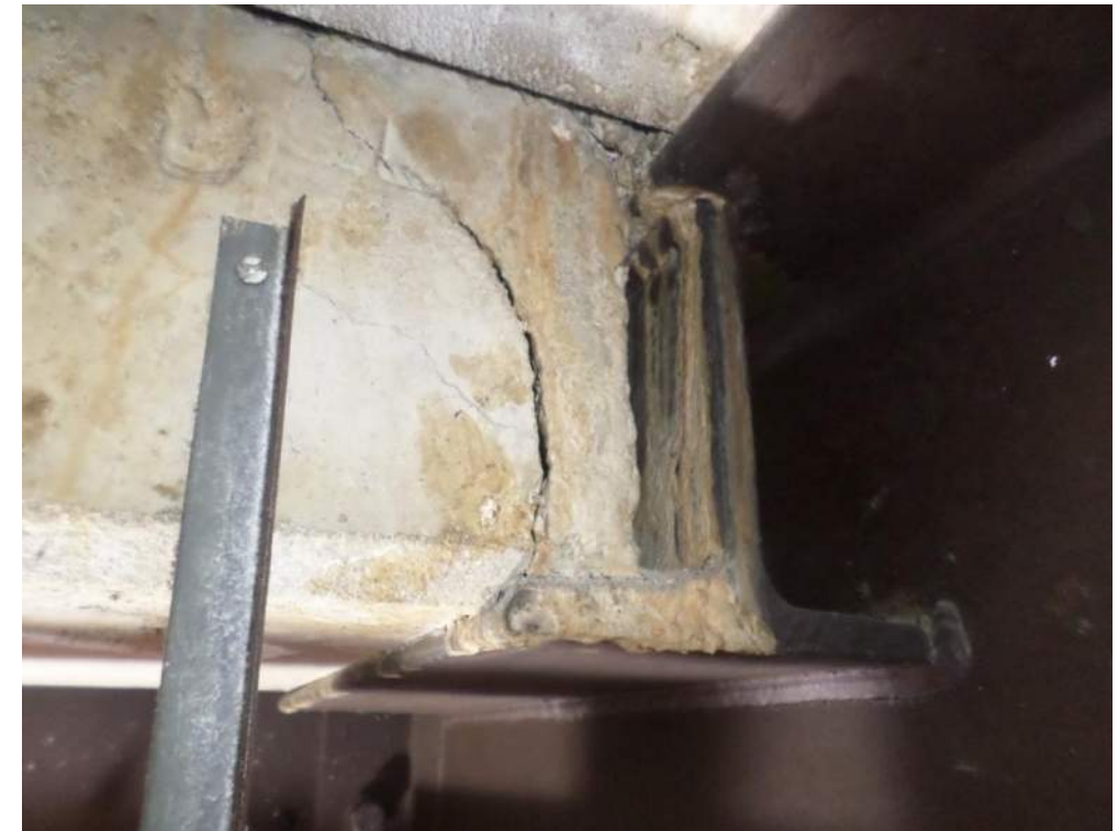
Shear failure of RAAC plank – NOT ST DAVIDS HALL
